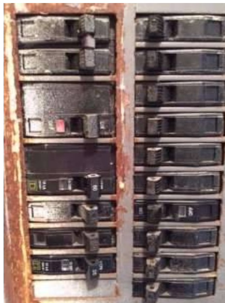
Photo 6-8 View of service panel.
