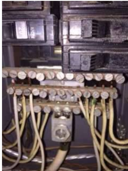
Photo 6-6 View of service panel.
