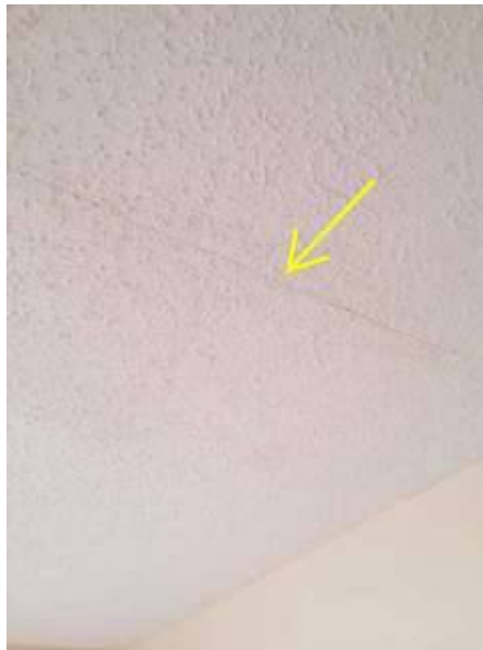
Photo X-8 Minor Tape Separation in Ceiling.
