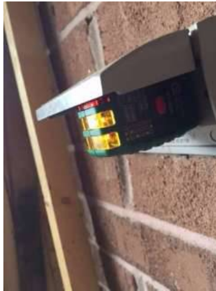
Photo X-30 Exterior GFCI receptacle in working order.
