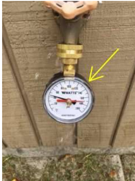
Photo X-10 Water pressure at rear Water Bib.
