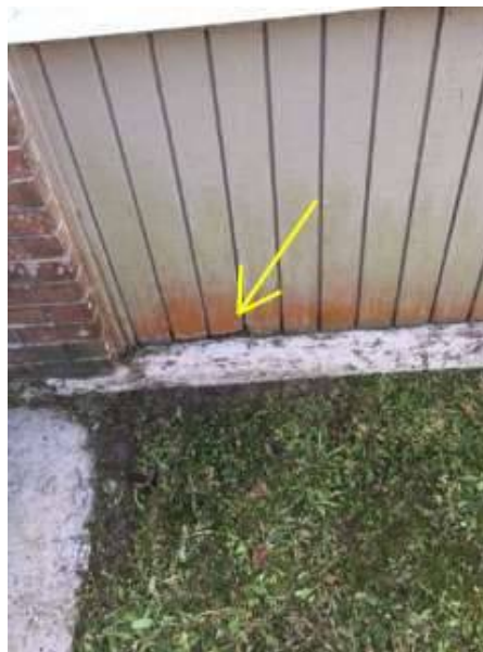
Photo X-12 Evident wood decay at base of exterior wall covering at screened porch.
