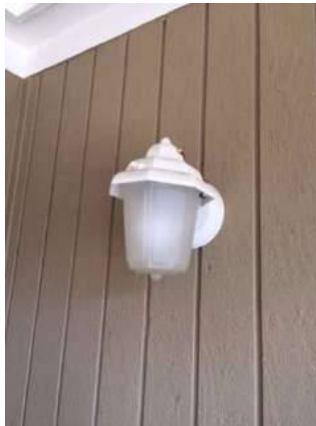
Photo X-32 Front light not operational - bulb replacement or repair.
