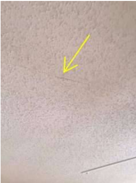
Photo X-9 Minor Tape Separation in Ceiling.
