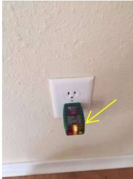
Photo 4-2 Open Ground - Inspected in both Living Room and Bonus / Guest Bedrooms.
