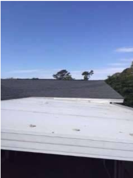
Photo X-17 View of Vinyl Roof Covering Back Porch- In working order and serviceable.
