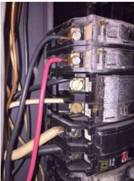
Photo 6-7 View of service panel.
