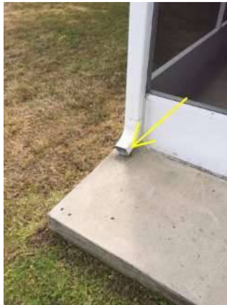
Photo X-24 Downspout should be extended beyond concrete.
