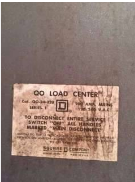
Photo 6-3 View of service panel.
