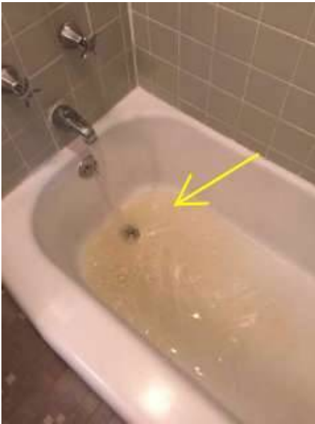
Photo 8-1 Discoloration of water supply.
