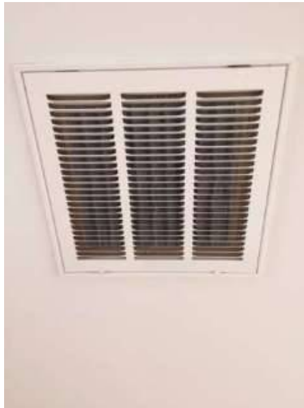
Photo X-6 Air Filter on Return - Bedroom.
