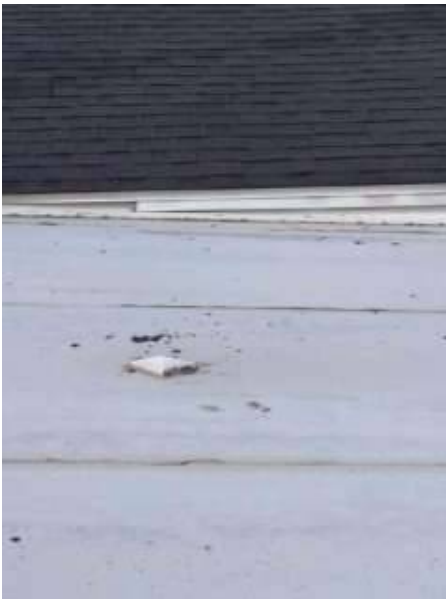
Photo X-19 View of Vinyl Roof Covering Back Porch- In working order and serviceable.
