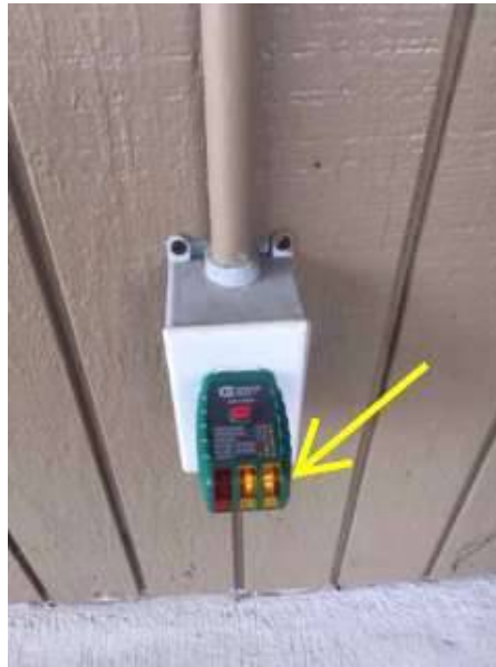
Photo X-26 Patio GFCI receptacle in working order.
