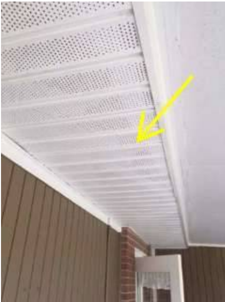
Photo X-25 Soffit vents in good working order.
