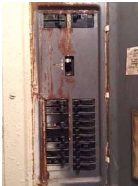
Photo 6-4 View of service panel.
