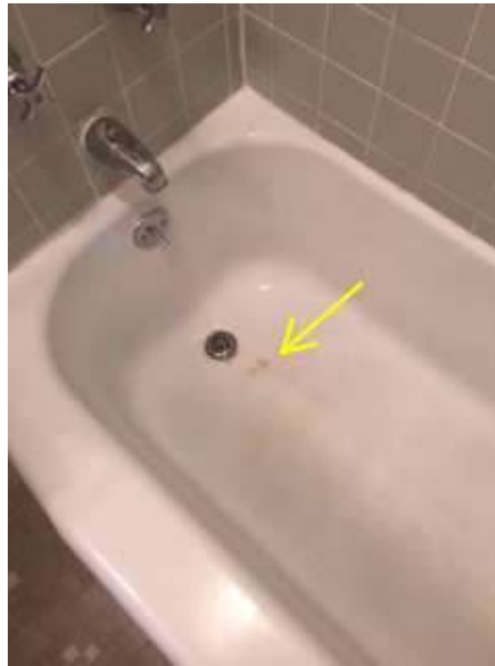
Photo 8-2 Sediment in water supply.
