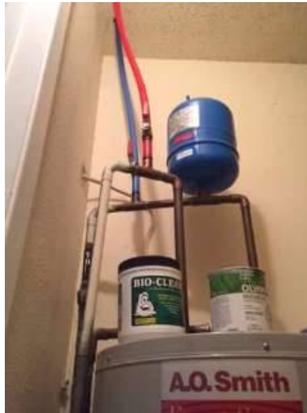
Photo 12-2 Expansion Tank - Water Heater.
