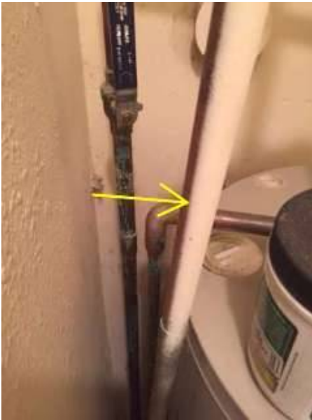
Photo X-33 Only visible area of non PVC piping with copper in place at water heater.
