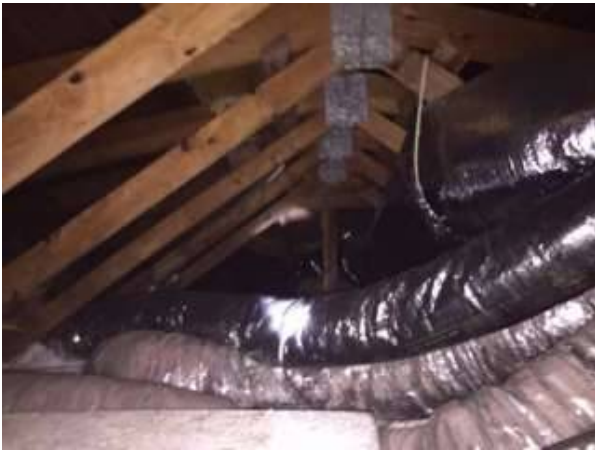
Photo X-5 View of attic duct work in working order.
