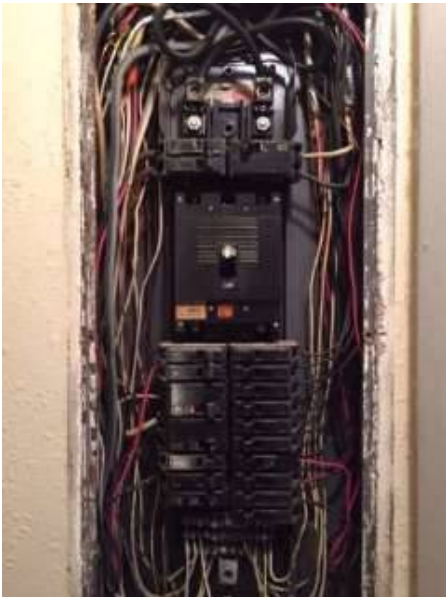
Photo 6-5 View of service panel.
