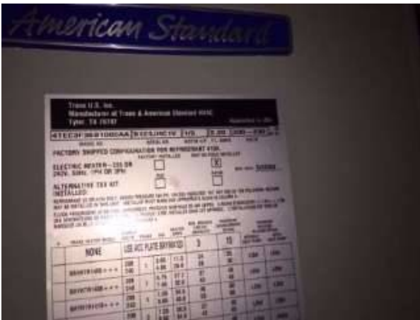
Photo 15-1 Manufacturers information on Air Handler in Attic. March 2009
