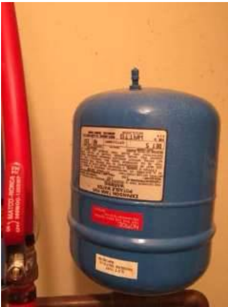
Photo 13-1 Expansion Tank - Water Heater.
