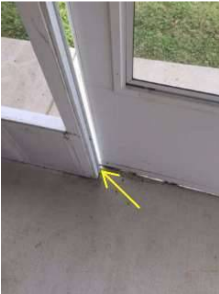
Photo X-21 Minor adjustment of rear patio door.
