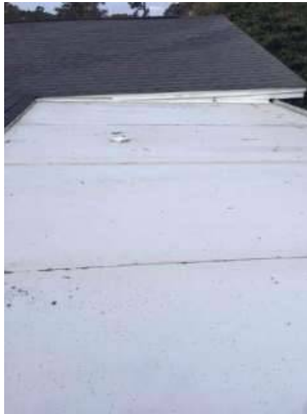
Photo X-18 View of Vinyl Roof Covering Back Porch- In working order and serviceable.
