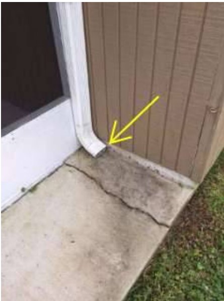
Photo X-23 Downspout should be extended beyond concrete.
