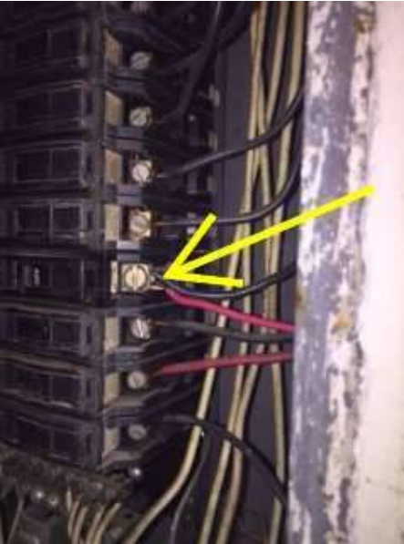
Photo 3-1 Suspected double tap inside service panel.
