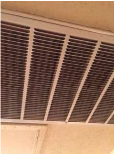
Photo X-7 Air Filter on Return- Utility Room.
