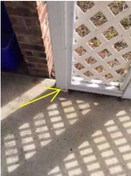
Photo X-13 Minor wood decay at lattice base in carport.
